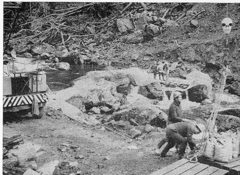
Work starting on the bridge over the Lyvia River which flows into Deep Cove
