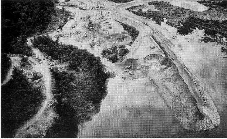
General view of servicing area at Deep Cove end of tailrace tunnel. Portal is at top left of photo
